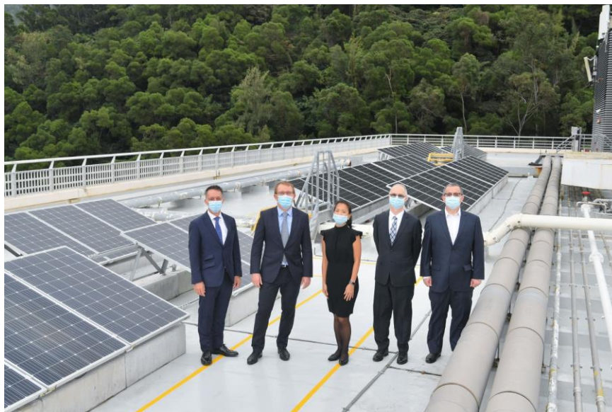
Luanne Lim, Chief Operating Officer, Hong Kong, HSBC (middle), Alex Keisser, Managing Director of CLPe Solutions (second from left) and senior representatives of the Bank visit the solar system at the rooftop of HSBC Building Tseung Kwan O.
